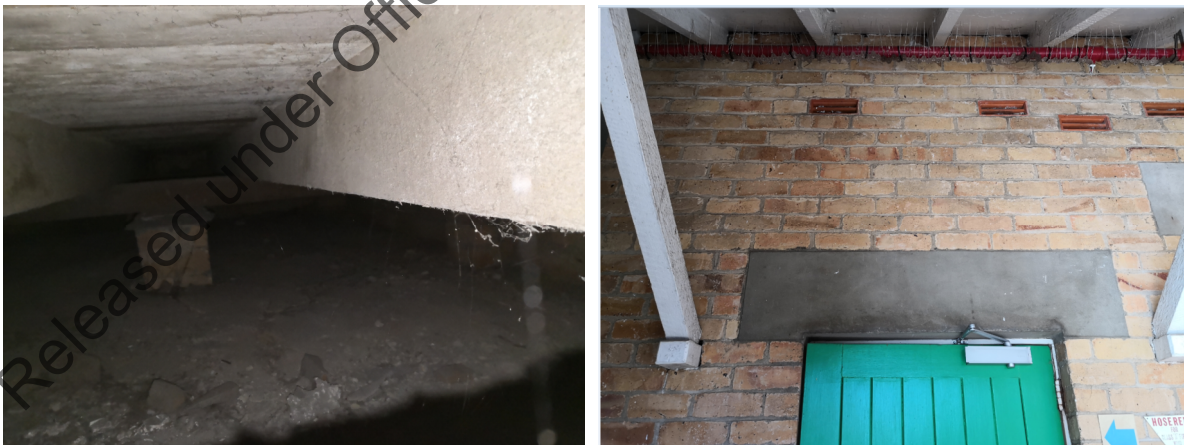
Figure 5: (left) Timber bearer sitting on solid brick column (right) concrete lintel above doorway
