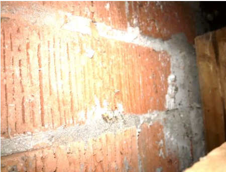
Concrete can be seen spilling out side of timber form
