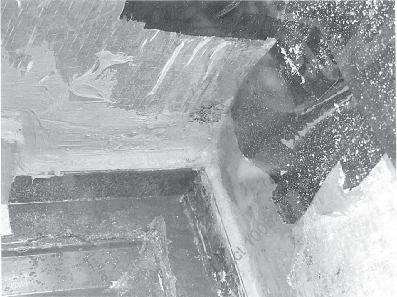
Figure 8 Uncontrolled water penetration through rear mitre joint. Evidence of oxidation damage to aluminium framing at mitre joints on both sides.
